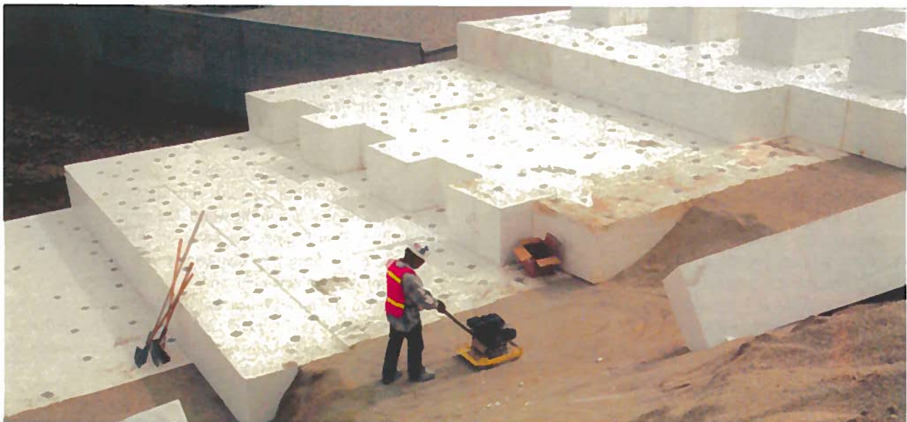
大约10万立方米的地基泡沫用在了可能发生沉降的地区 Around 100,000 cubic metres of geofoam was used in settlement prone areas
