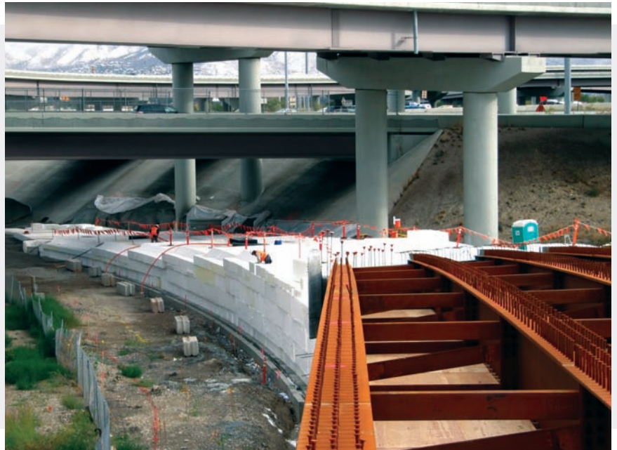
Seven areas along the West Valley TRAX line required the use ACH Foam Technologies' EPS geofoam.
