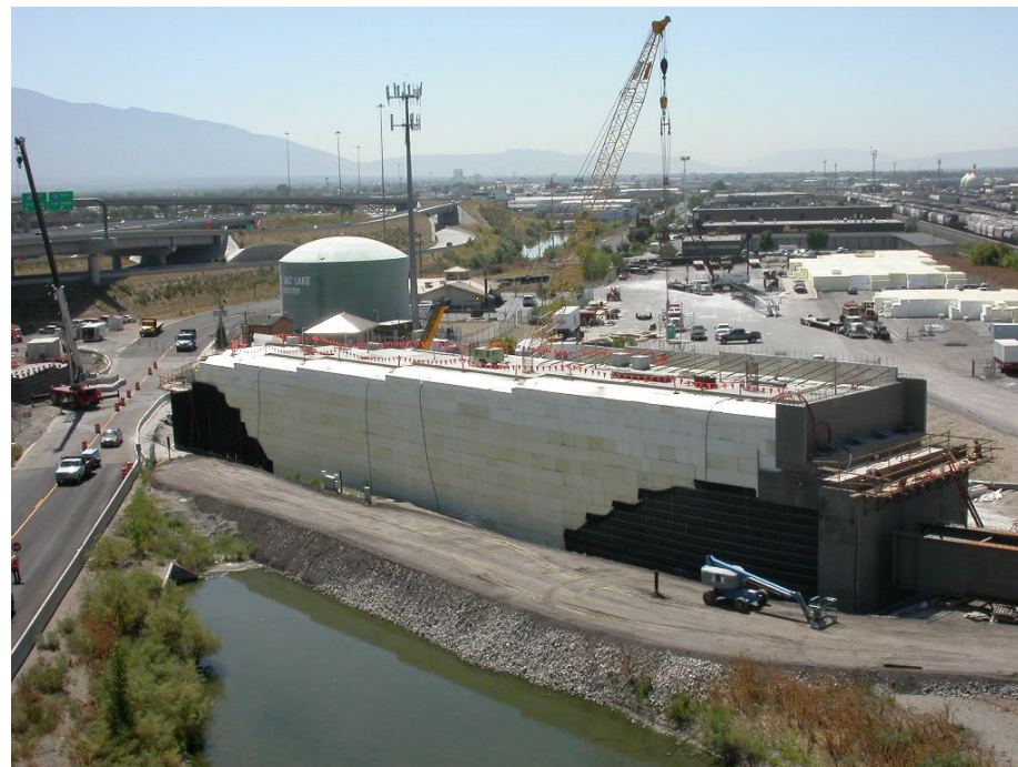
Geofoam embankment – Utah Transit Authority Light Rail System Salt Lake City, Utah
