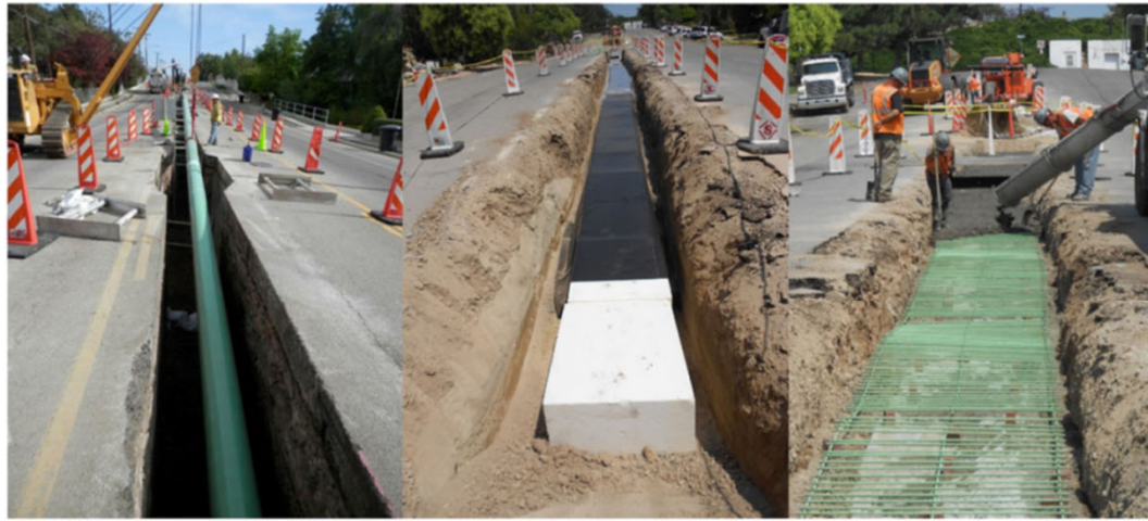
Fig. 5. EPS slot-trench light-weight cover system constructed across the Wasatch fault in Salt Lake City, Utah. Left photo is placement of 0.6-m diameter ductile steel pipe. Middle photo is placement of EPS geofoam and geomembrane cover. Right photo is construction of concrete load distribution slab before placement of roadway section.
