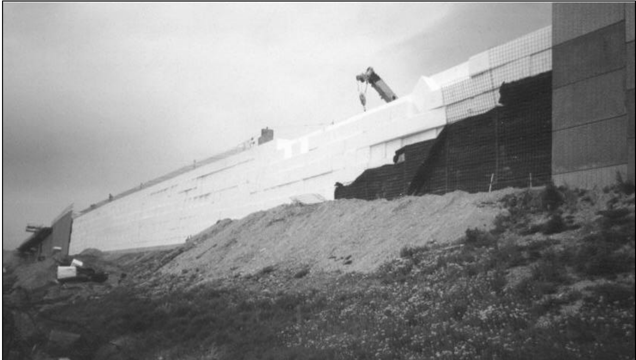
Figure 4. Geoforembankment construction near the 3300 South Street Northbound off ramp. The far end (i.e., south) of the geoforembankment has been placed against the abutment of the Union Pacific Overpass. The closest end (i.e., north ends) transitions into a MSE wall. Tilt-up wall panel placement has begun on the south end of the embankment.
