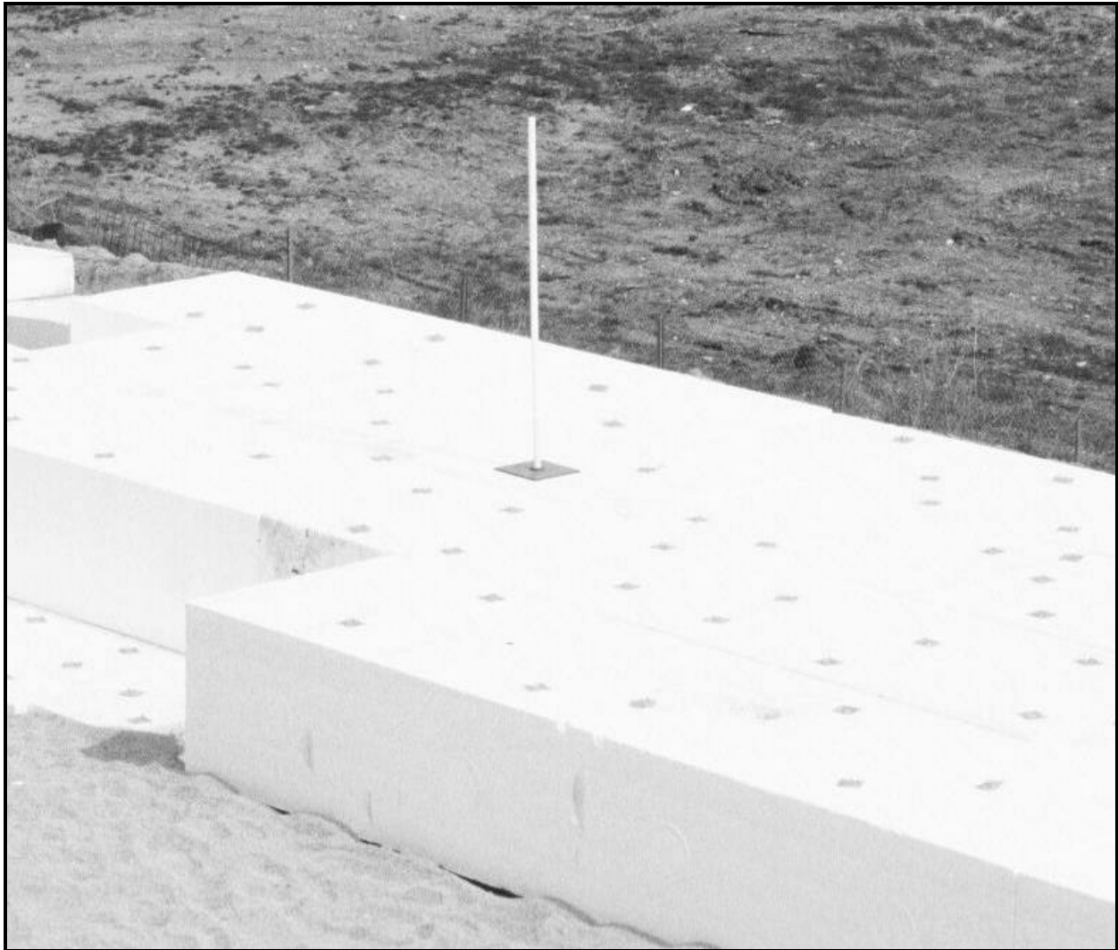
Figure 8. Magnet extensometer installation within the geofabric embankment. Note the plastic plate with ring magnet has been placed atop the geofabric block. The plate is subsequently covered by additional geofabric layers.
