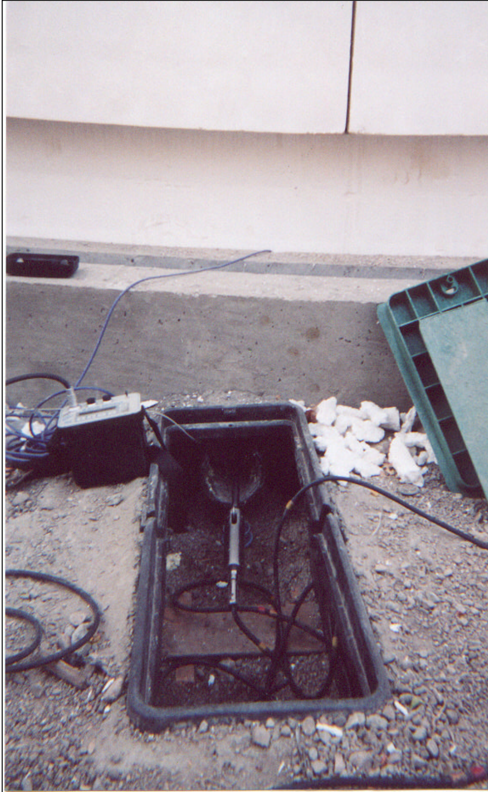
Figure 6 – Access port for the north array basal inclinometer beneath the fascia wall grade beam (See Figure 3).
