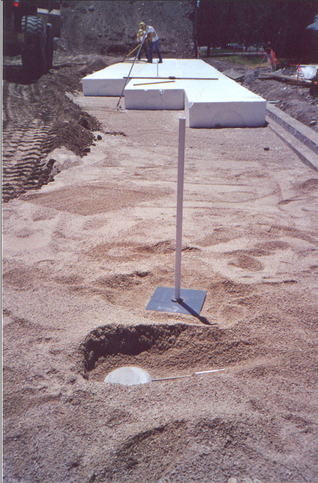
Figure 4 – Stress cell and extensometer plate in the leveling course below the geofilm fill. Note geofilm and grade beam for fascia wall support in background.
