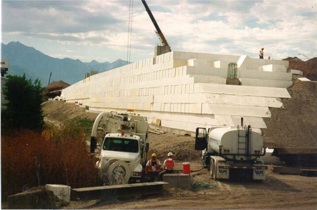
Figure 1. Typical geofabric embankment construction on the I-15 Reconstruction Project in Salt Lake City, Utah.
