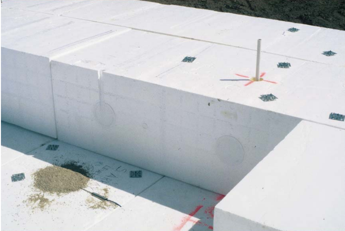
Figure 3. Geofoam array at 3300 South south array, showing a concealed pressure cell, PVC riser pipe, and gaps between block layers.
