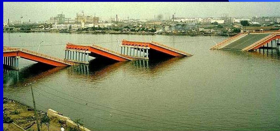
1964 Niigata, Japan Earthquake
