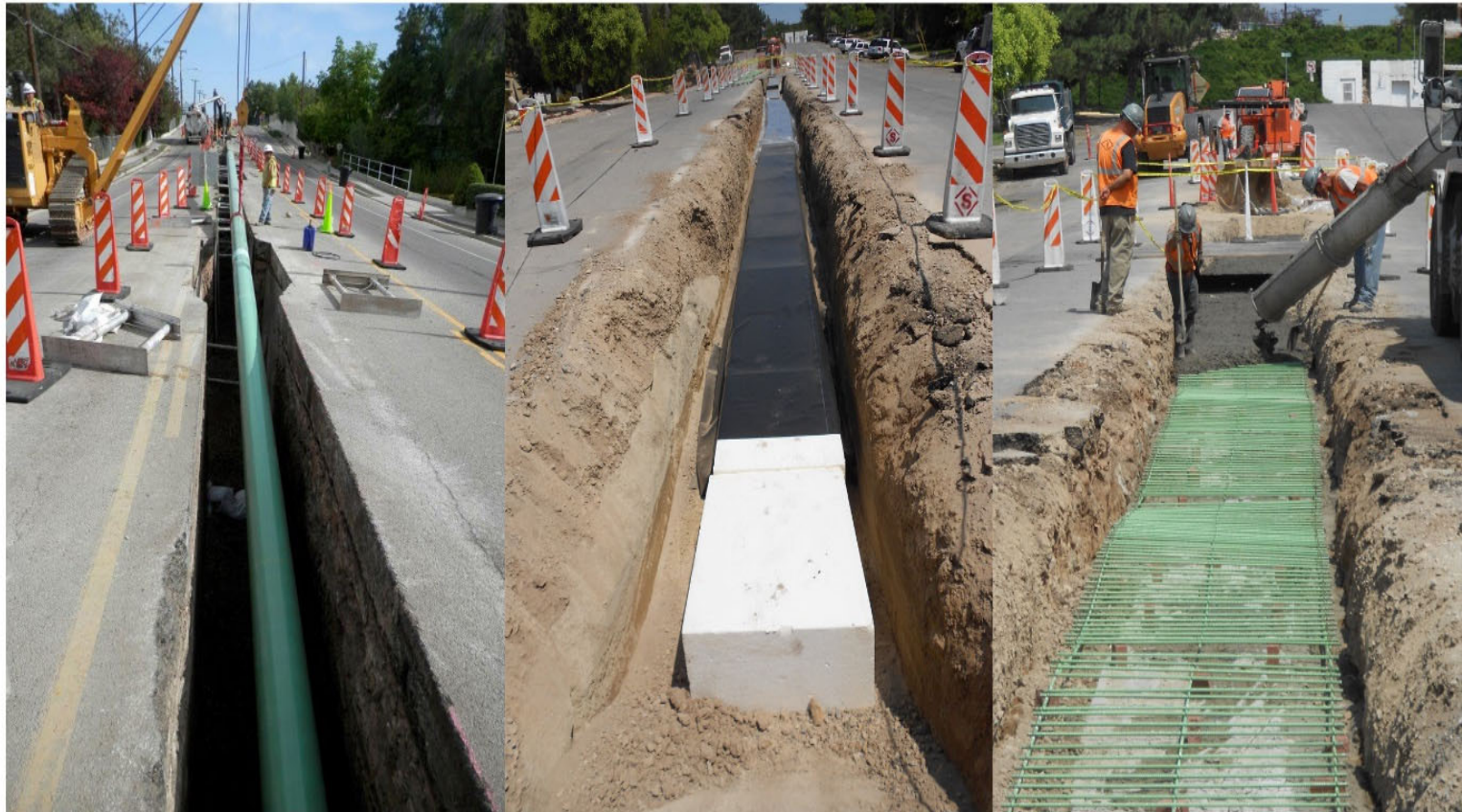
Crossing of Wasatch Fault Zone in with High-Pressure Gas Line Salt Lake City, Utah, Questar Gas Corp.
