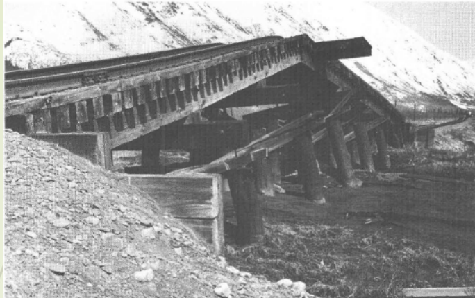
Jack-Knifed Bridge due to Compression
