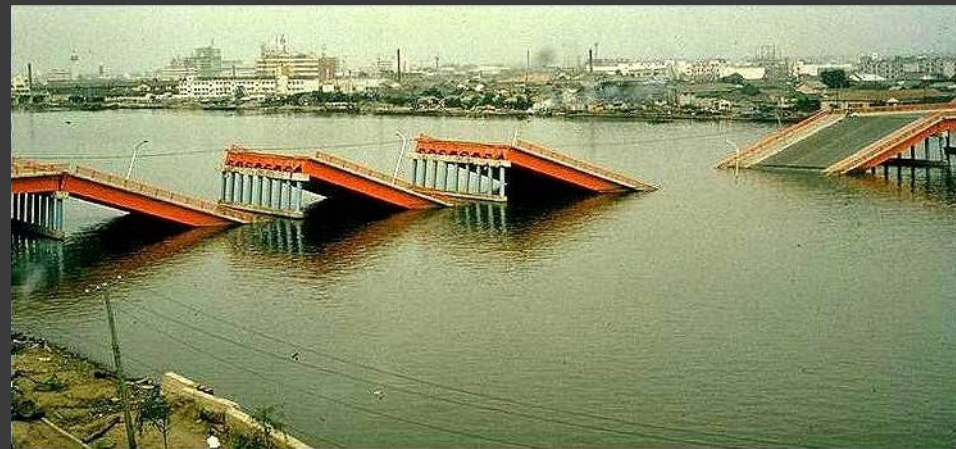
1964 Niigata, Japan Earthquake
