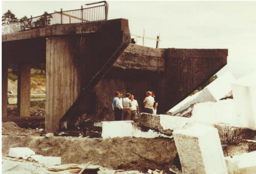
Fig 34. Bridge abutment damaged by EPS blocks put on fire
