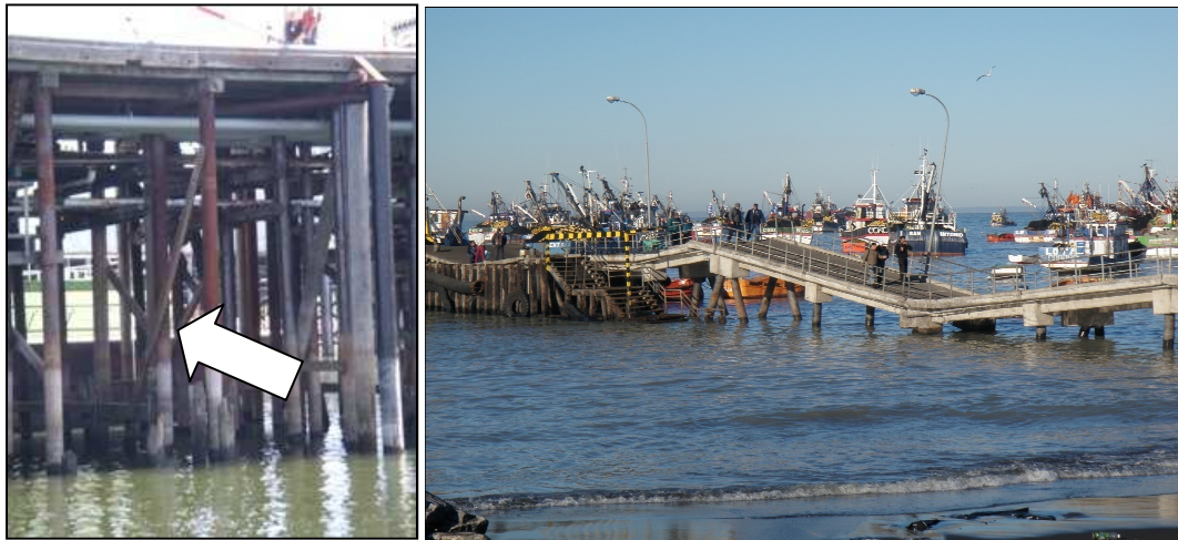
Left: Lateral timber bracing for steel plumb piles in the CEI Hub is considered inadequate by California's MOTEMS standards. (DOGAMI photo) Right: An example of a damaged pier in the 2010 Chile earthquake (Technical Council on Lifeline Earthquake Engineering – TCLEE, 2010)
