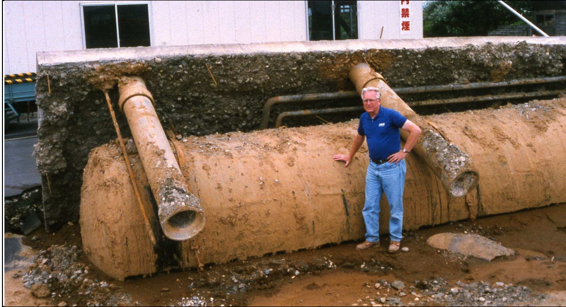
Figure 18: Buried tank in liquefied soil that was uplifted due to buoyancy forces in the 1993 Hokkaido-Nansei-Oki Earthquake and Tsunami in Japan (Photo permission on 1/9/12 from Youd; Youd, T.L. et al 1995, Photo taken by R. Chung)
