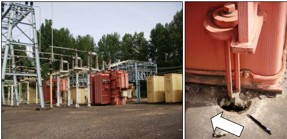
Figures 68 and 69: The photo on the left shows high voltage transformers (orange color) in the CEI Hub that require proper anchorage. The close-up photo on the right shows that the transformer is anchored, but the anchorage was poorly installed or poorly maintained as evidenced by the amount of grout that is missing. (DOGAMI photos)
