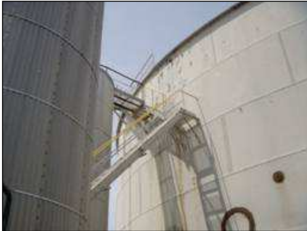
Figure 63: The elements connecting the tops of these two tanks in the CEI Hub may cause damage to the tanks during shaking due to differential displacements. (DOGAMI photo)
