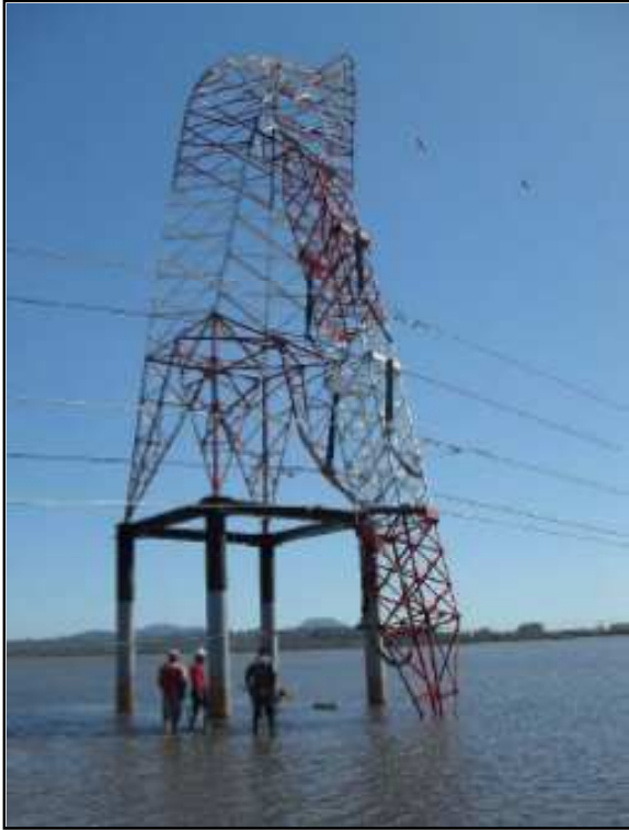
Figure 60: Structural damage to high voltage transmission tower located in river crossing in 2010 Chile earthquake. This limited electricity availability while temporary towers were installed (Technical Council on Lifeline Earthquake Engineering - TCLEE)
