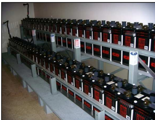
Emergency batteries, as well as other components such as generators and communication devices, should be braced or anchored to withstand Cascadia earthquake. (DOGAMI photo)
