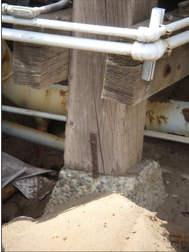
Figure 36: This under-designed foundation in part of an oil terminal pier in the CEI Hub is considered inadequate. Based on previous regional studies, boring logs from an adjacent facility, and on-site visual inspection of the surficial soils, this area has high susceptibility for liquefaction and lateral spreading. (DOGAMI photo)
