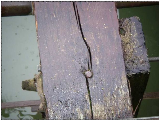
Figure 41: The connection on this pier in the CEI Hub appears to have deteriorated due to a split in the timber beam. This type of damage suggests that the condition of the structure may not be routinely monitored and maintained and that the overall pier is seismically vulnerable. (DOGAMI photo)
