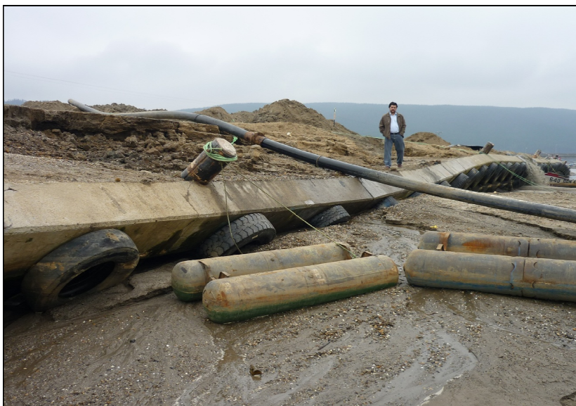
Figure 23: Lateral spreading damage from the 2010 magnitude 8.8 Chile earthquake. (Technical Council on Lifeline Earthquake Engineering - TCLEE)
