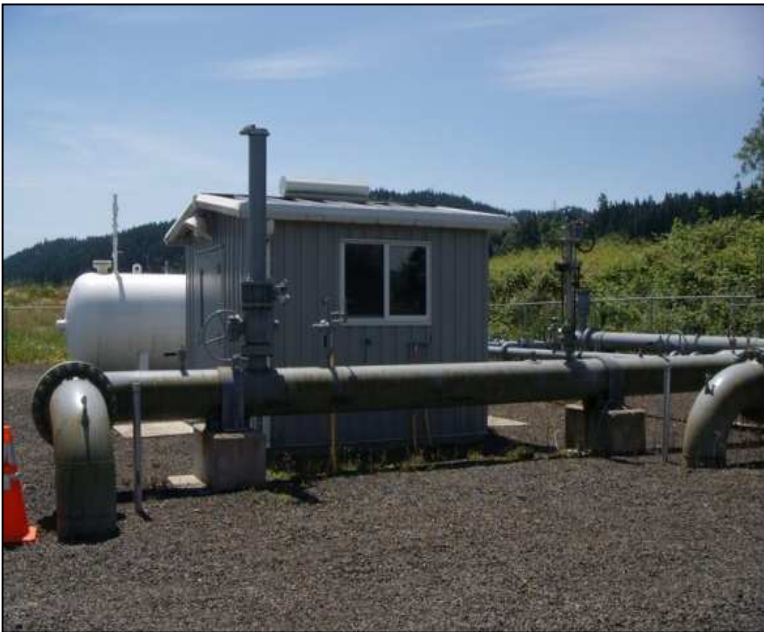
Figure 53: Several liquid fuel and buried natural gas pipelines at the Columbia River and Willamette River crossings just north of the CEI Hub. Photo shows a natural gas gate station on Sauvie Island. (DOGAMI photo)
