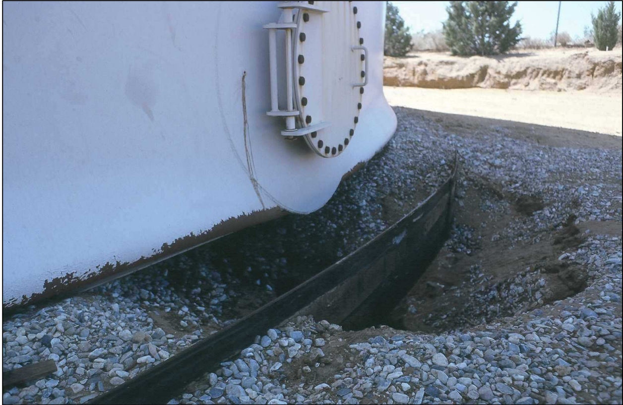
Figure 26: Welded steel water tank damaged in 1992 Landers, California earthquake. (Photo - Curt Edwards, Technical Council on Lifeline Earthquake Engineering - TCLEE)
