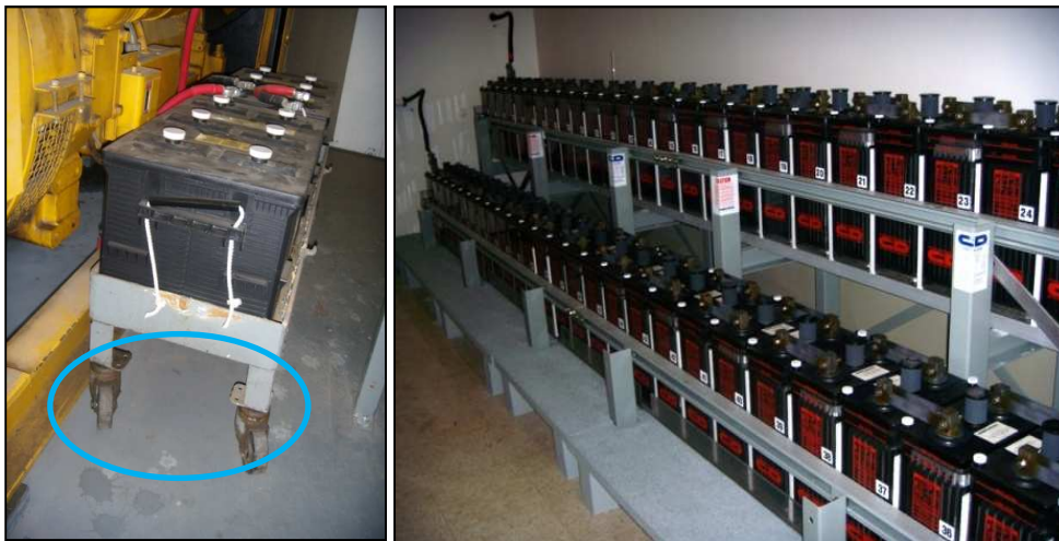
Figures 64 and 65: Batteries should not be on a wheeled cart as in the photo on the left. Emergency batteries, as well as other components such as generators and communication devices, should be braced on an anchored rack to withstand Cascadia earthquake forces as in the photo on the right. (DOGAMI photos)
