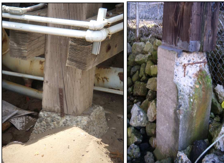
This under-designed oil terminal pier foundation (left) in area with high susceptibility for liquefaction and lateral spreading in the CEI Hub and the poor timber-to-concrete oil terminal pier connection and exposed rebar foundation (right) in the CEI Hub are considered inadequate. (DOGAMI photo)
