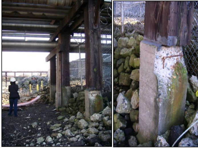
Figures 39 and 40: The close-up photo on the right shows poor timber-to-concrete connection, broken concrete and exposed rebar. Energy sector companies should maintain and upgrade infrastructure to current standards in order to protect assets and limit down-time following an earthquake. (DOGAMI photos)
