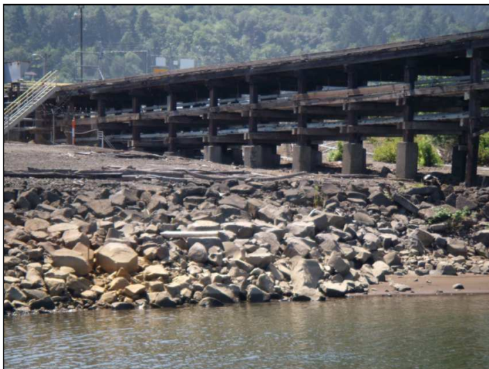
Figure 37: The area by this pier in the CEI Hub is used to transport liquid fuel. Based on previous regional studies, boring logs from an adjacent facility, and on-site visual inspection of the surficial soils, this area has high susceptibility for liquefaction and lateral spreading. (DOGAMI photo)
