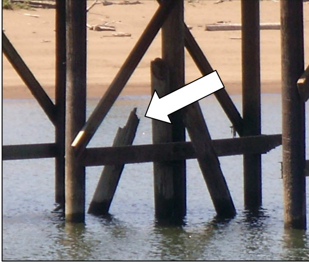
Figure 42: This pier in the CEI Hub appears to be poorly maintained with broken timber piles adjacent to working components of the pier. (DOGAMI photo)
