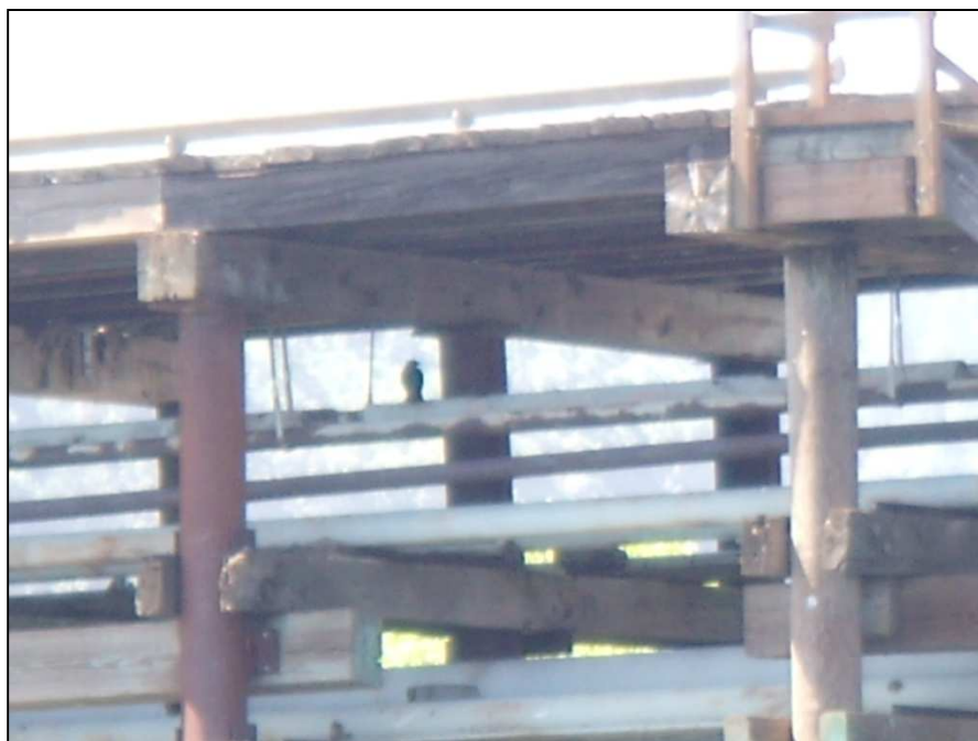
Figure 38: This photo shows generally poor condition of transverse beams supporting petroleum pipelines and cap beam in the CEI Hub. Notice the clockwise rotation of the pile cap beam in the center of the photo. (DOGAMI photo)
